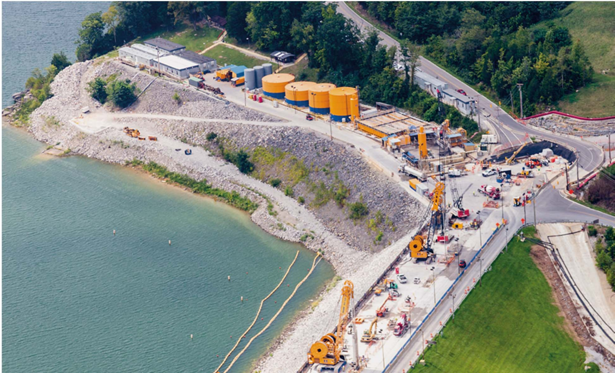
Figure 1. BAUER MC 128 (left) and MC 96 (right), both equipped with hydrocutters, working during barrier wall installation
