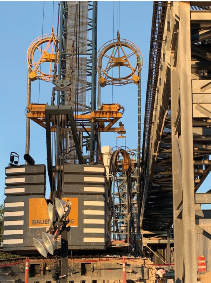
Cutter working in close proximity to a conveyor belt
