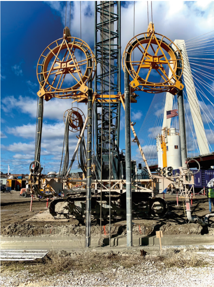
Cutter excavating bedrock at the upstream end of the project (Stan Musial Bridge in the background)
