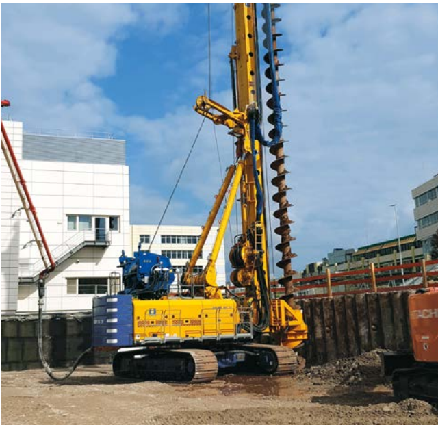
New building of central laboratory, Herzogenaurach, Germany Drilling of foundation piles with a diameter of 1,000 mm and depth of 18 m using the CFA method.
