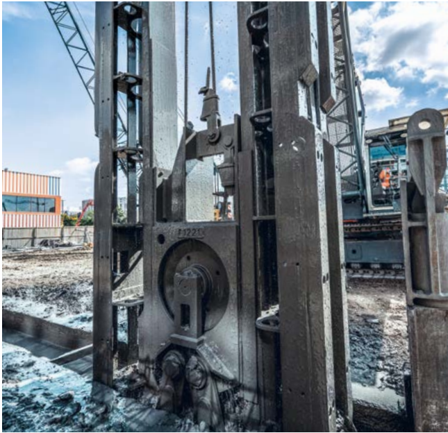
South entrance to exhibition grounds, Frankfurt am Main, Germany Execution of a 2-phase diaphragm wall using an MC 64 duty-cycle crane with grab.
