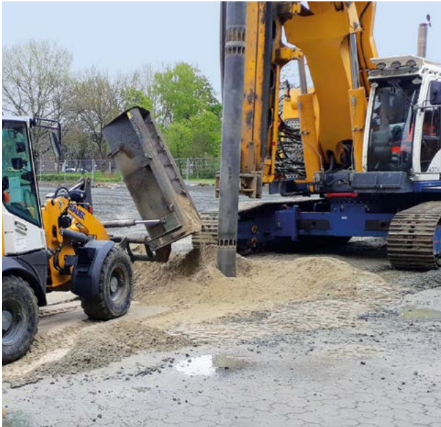
Center for Deep-Sea Research (Zentrum für Tiefseeforschung – ZfT), Bremen, Germany For the new ZfT building in Bremen, Bauer executed 5,500 m of vibro compaction work.
