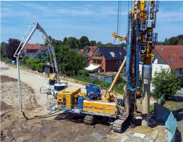
Businesspark, Hannover, Germany Construction of secant pile wall with a diameter of 880 mm and depth of 16 m using the double-head drilling method.
