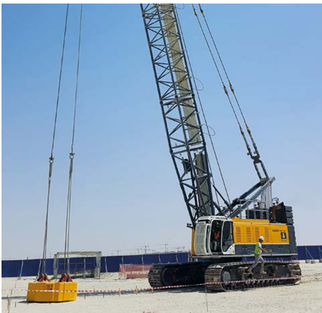
Dubai Creek Harbor, Dubai, UAE Improvement of the construction soil over roughly 500,000 m 2 using vibro compaction and dynamic compaction.
