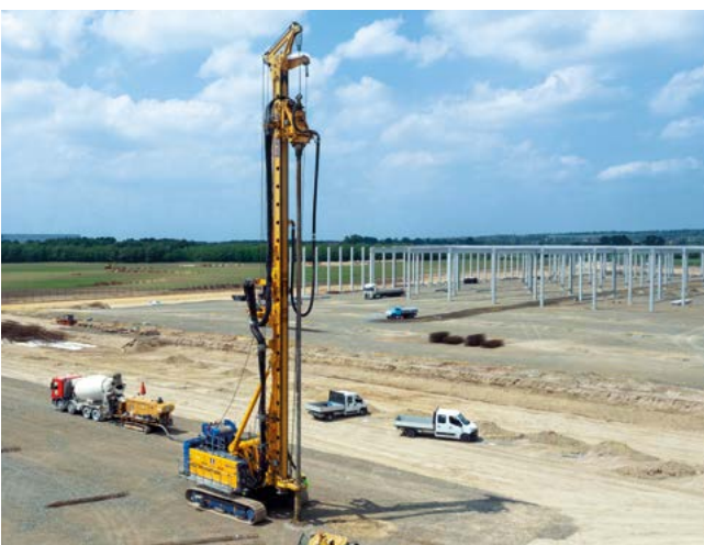
New construction of logistics halls, Maglód, Hungary Construction of foundation piles with a diameter of 360 mm using FDP method.
