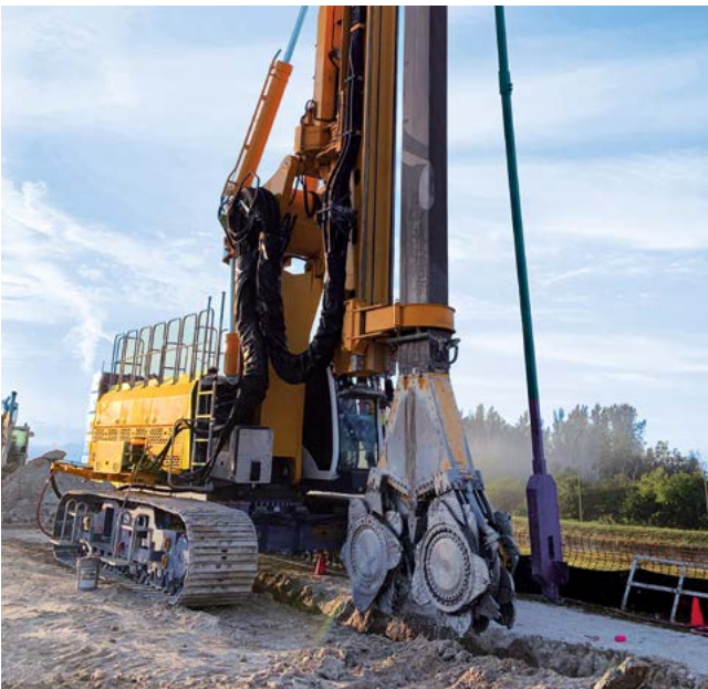
Herbert Hoover Dike, Florida, USA To improve dam security, a 28.3 km cut-off wall was installed with a depth of up to 20 m.
